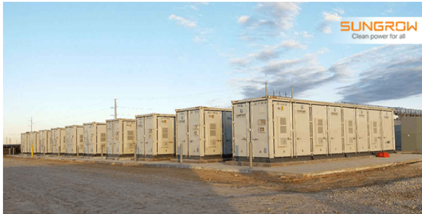
TYPICAL SUNGROW ENERGY STORAGE CONTAINERS
