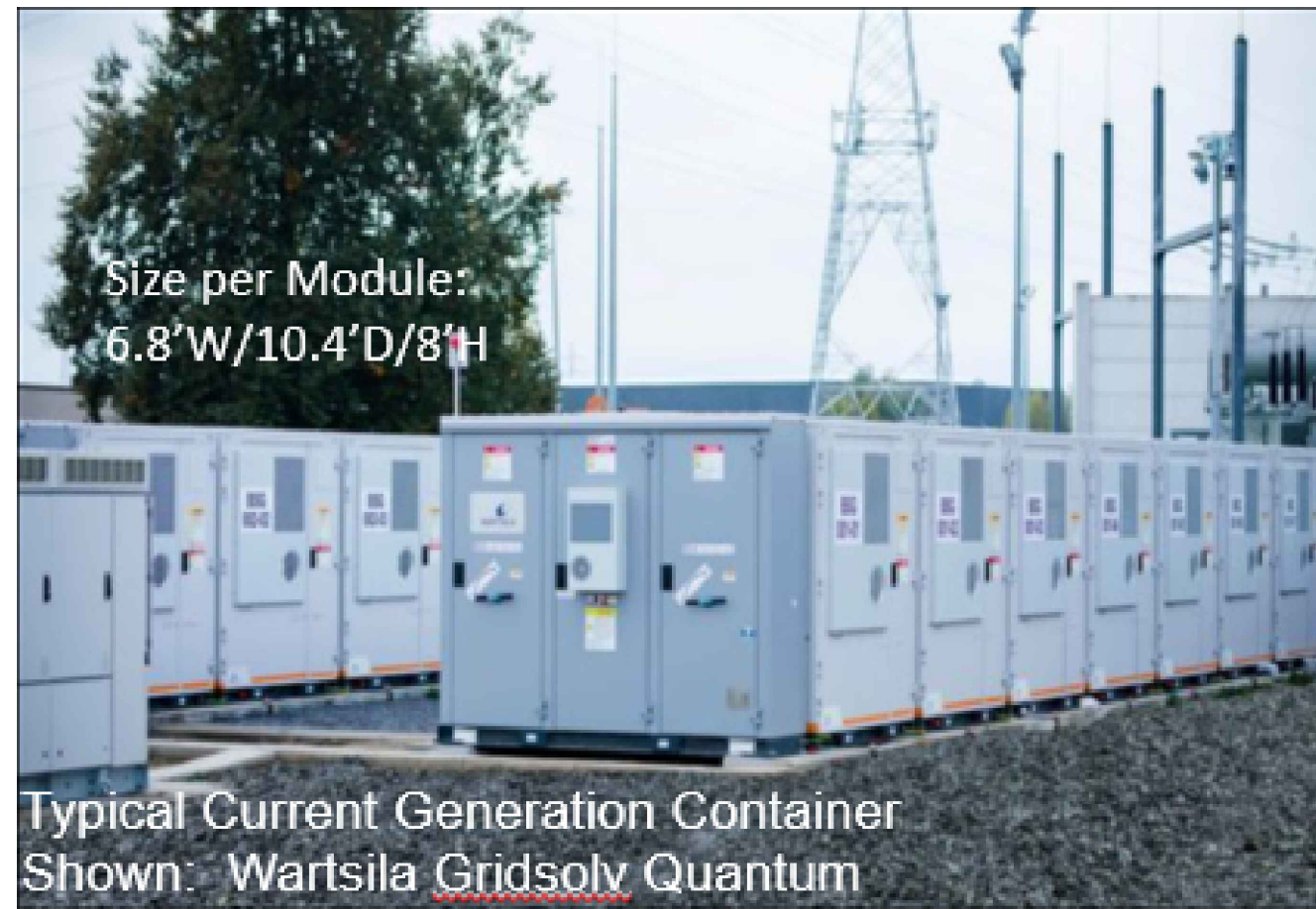
TYPICAL WARTSILA ENERGY STORAGE CONTAINERS
